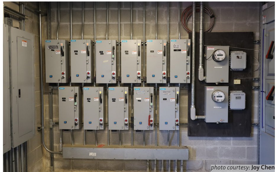
PHS energy meters keep track of electricity usage in the school. In the last week of May, PHS used 69,420 kWh of energy, over double the national average.
